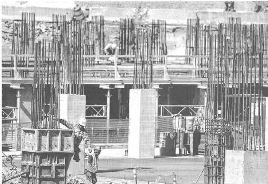
Geotechnical consultants TTL take samples of all the concrete poured during construction of the Music City Center to test for durability and adherence to specifications. More than 30,000 cubic yards of concrete have been poured, with an additional 80,000 estimated to complete the project. TTL samples concrete every 50-75 yards. SAMUEL M. SIMPKINS / THE TENNESSEAN
